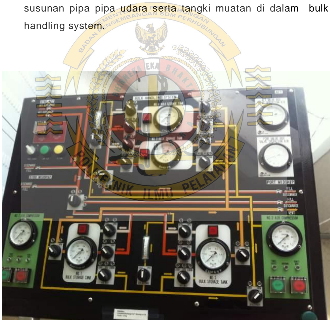
Gambar 1.1: Panel switch board bulk handling system
