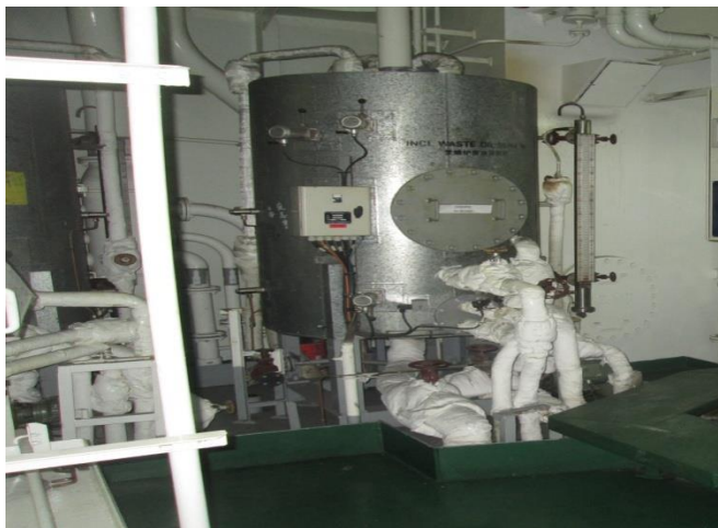
Gambar2. 5 Waste oil tank
