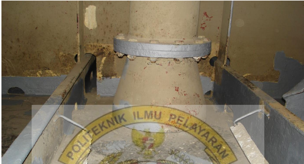
Gambar: Pipa Input & Output Air Ballast
