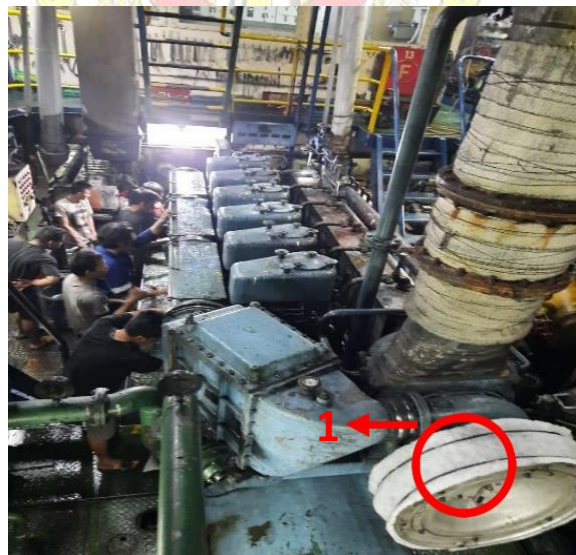
Gambar 4.8. Filter udara turbocharger sesudah diganti
