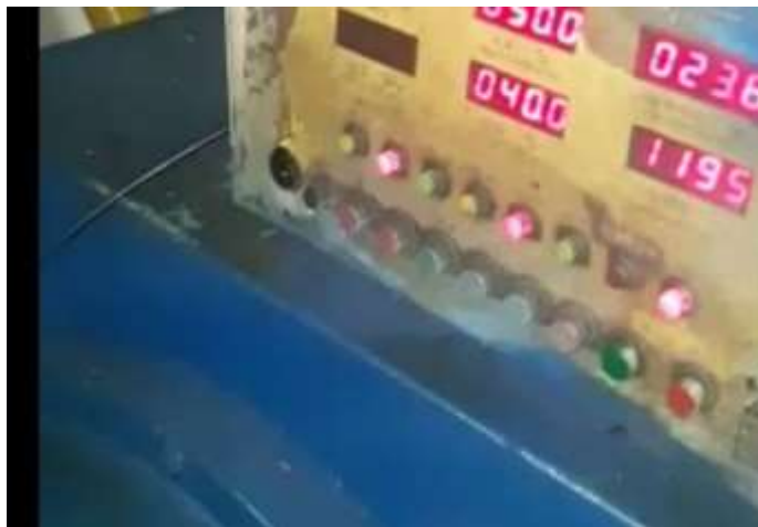
Gambar. Panel Box Diesel Generator
