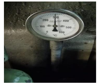
Sumber. Dokumentasi pribadi Gambar. 4.4 Thermometer Exhaust Gas Diesel Generator
