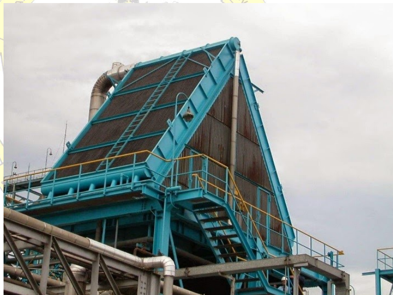
Gambar 2.12 Air Cooled Condenser
