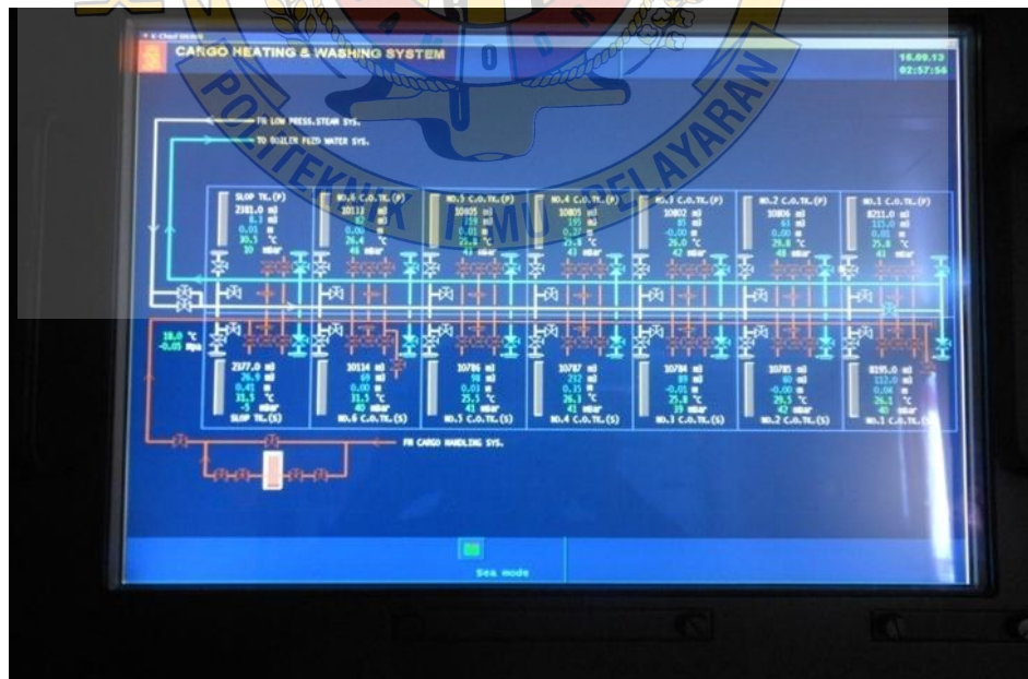
Gambar 4.2 Monitor CCR crude oil washing
