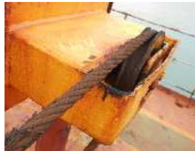
Gambar 2. Block wire hatch cover
