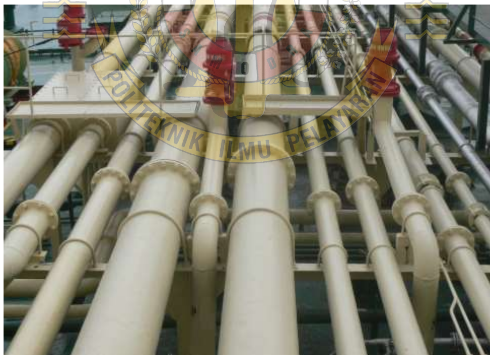
Gambar 5.4 Pipe Line Cargo
