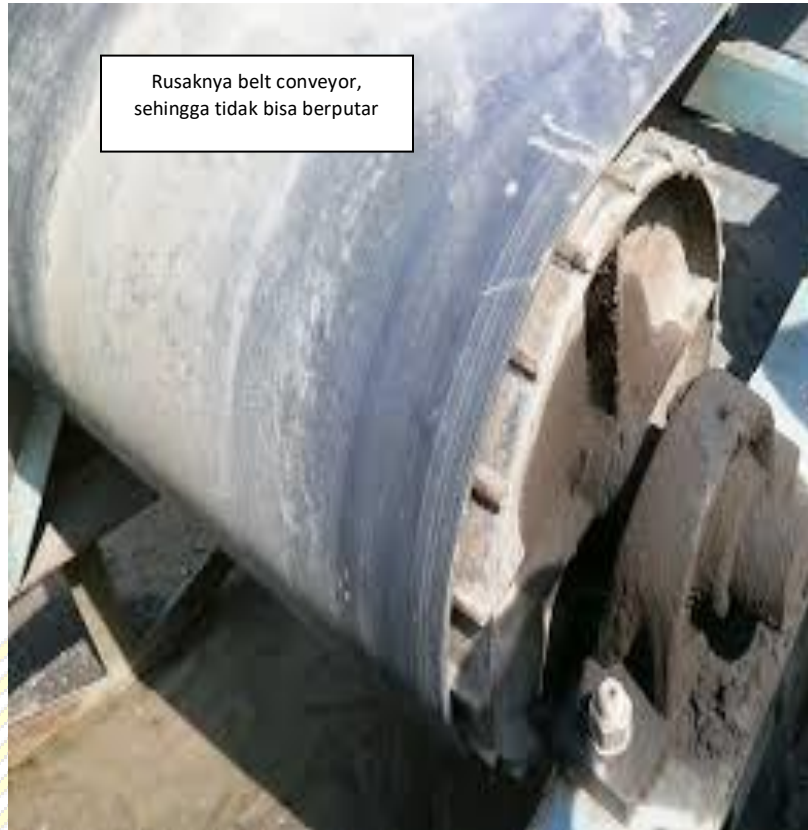
Gambar kerusakan conveyer
