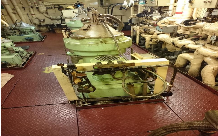
Unit Fuel Oil Purifier
