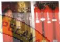
Fig. 7.6.3-1 CO2 Fixed Fire Extinguisher
