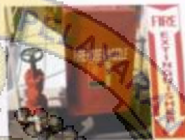
Fig. 7.6-3 Fire Hose and Nozzle with Fire Hydrant
