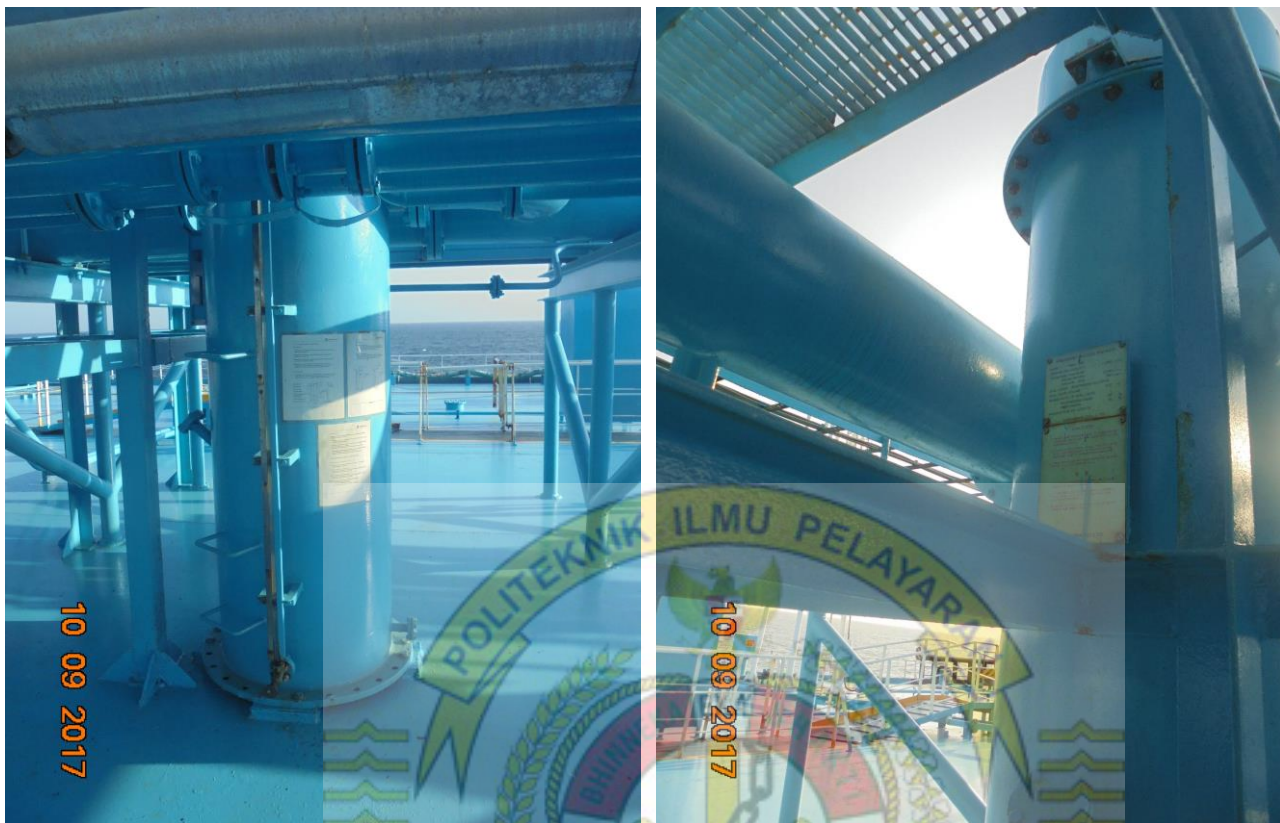
Gambar 3 : Pressure / Vacum Breaker (MT. GEDE)
