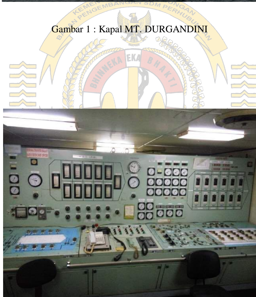
Gambar 2 : Cargo Control Room MT. DURGANDINI
