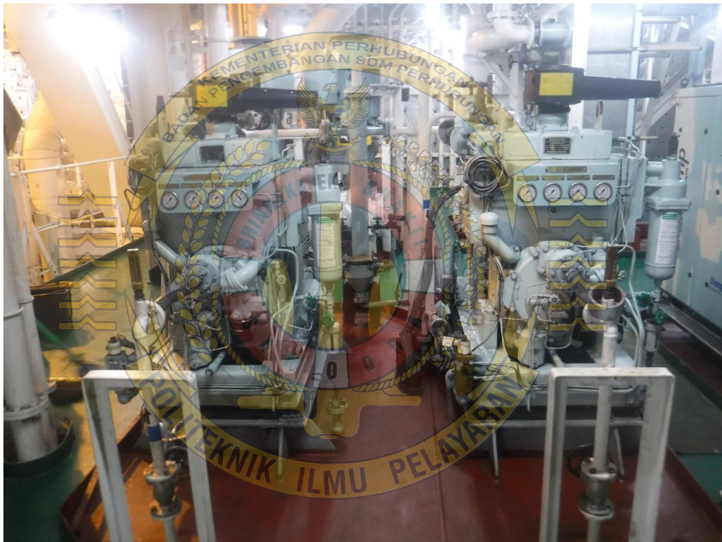
Main Air Compressor
