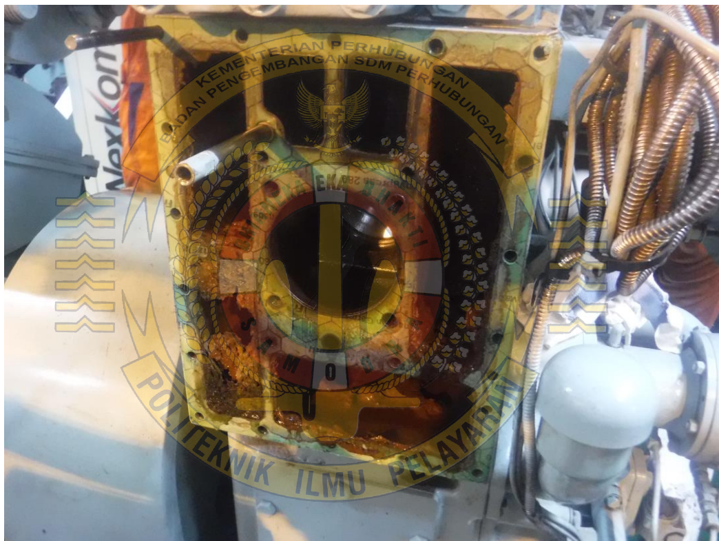
Packing Jacket cooling Main Air Compressor kondisi rusak Sumber data: Dokumentasi Engine Room MV. Ultra Alpha
