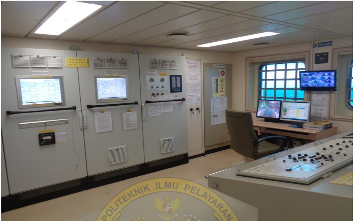
Gambar Cargo Control Room (CCR)
