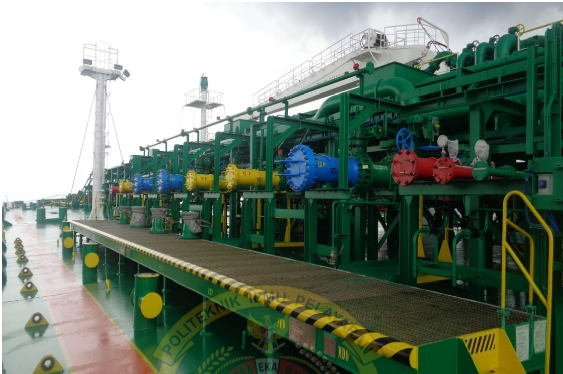
Gambar Manifold VLGC Pertamina Gas 2
