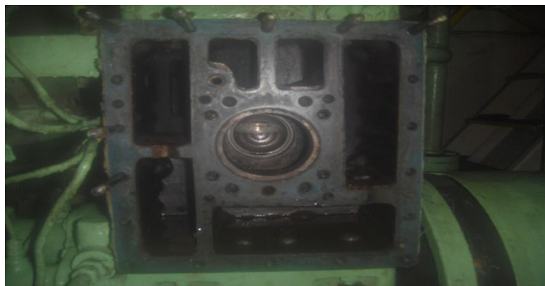
Gambar . 2.2 Jacket Cooling Main Air Compressor
