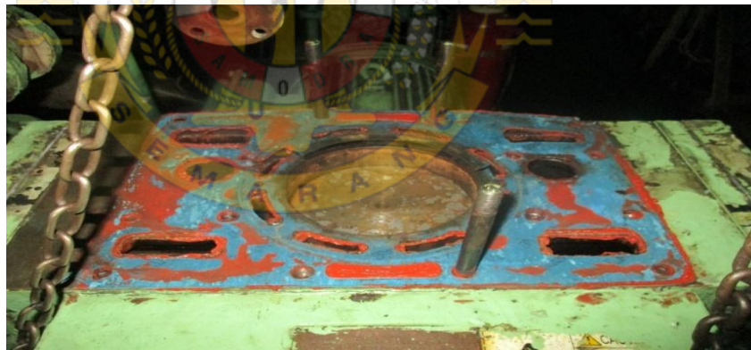
Gambar 2.5. Cylinder liner main air compressor
