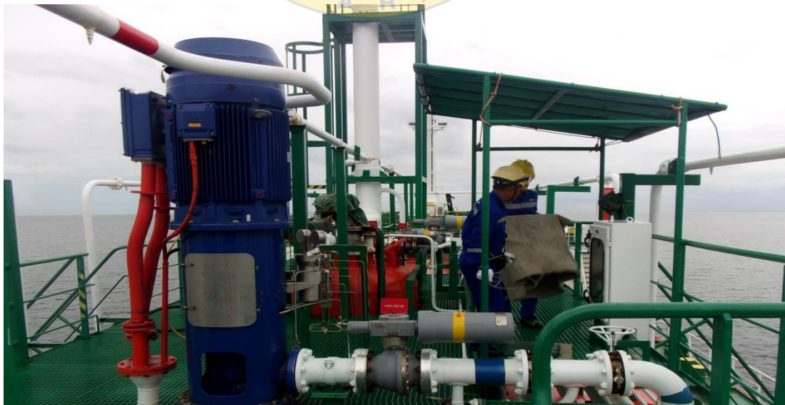
Gambar 5.3 Cargo pump Kapal Gas Arar
