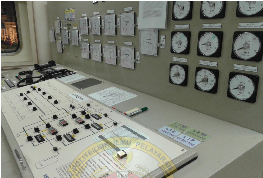
Gambar 5.10 Ballast Control Monitor Kapal Gas Arar
